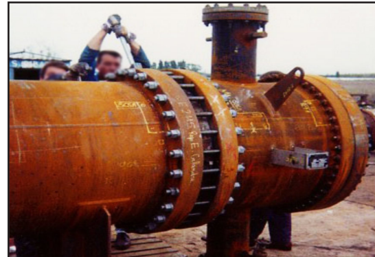
Re-assembly with Chesterton 785 Parting Lubricant stops corrosion and seizure.
