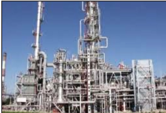
Scheduled PM outages every 24 months on heat exchangers requires complete disassembly.
